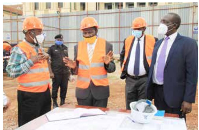
The Minister of Finance, Planning and Economic Development, Hon. Matia Kasaija being briefed by the Permanent Secretary and Secretary to the Judiciary on the progress of the construction.
