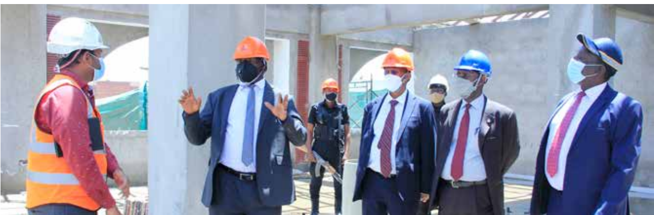
Members of the Judiciary Top Management led by the Chief Justice, Alfonse Chigamoy Owiny - Dollo inspected at its different construction stages.
